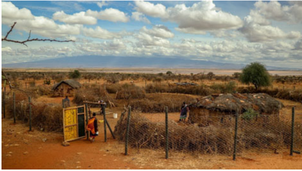
PLATE 1 A predator-proof boma under construction by the Born Free Foundation's Pride of Amboseli programme in 2018 ( Acacia thorn bushes have not yet been added to the outside perimeter).
